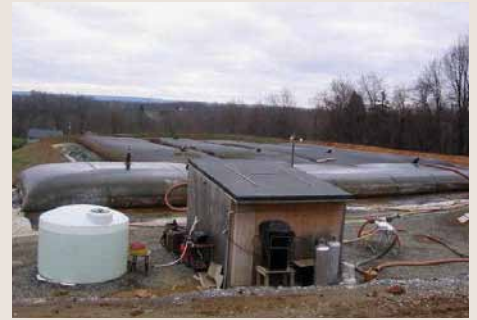
Geotube® dewatering cell
