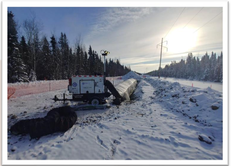
A single CH12MS heater heating a large section of a pipeline in winter conditions
