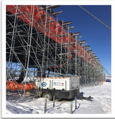
A CH15MS heater curing a large concrete section on a construction project
