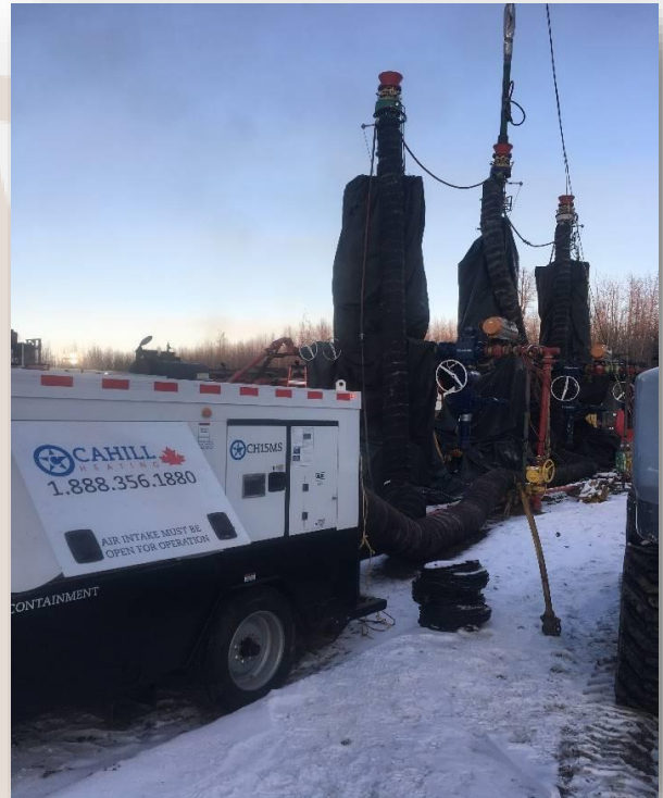
A CH15MS heater heating multiple BOPs simultaneously using split ducting on an oilfield
